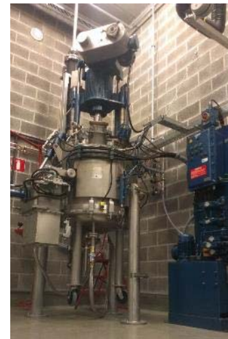
400L maceration plant
